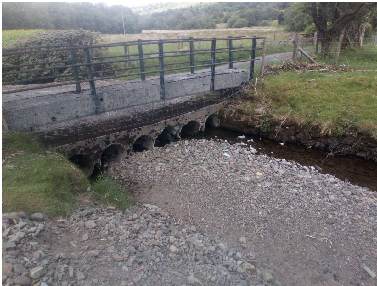
FIGURE 4.2: THE ACCUMULATION OF SEDIMENT UPSTREAM OF THE TYLE-Y-GARW CULVERT, HEOL SENNI.
